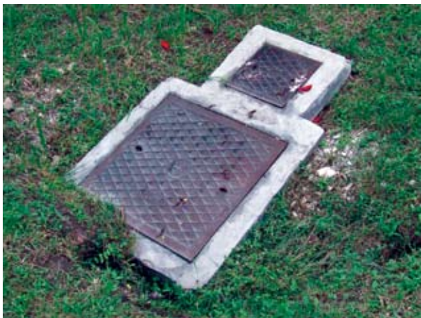
An intact manhole cover that has so far escaped theft.
