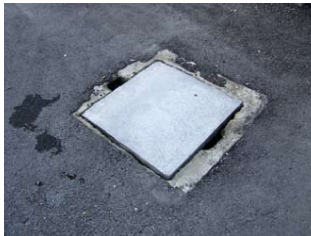
A stolen cover replaced by a cement replica
