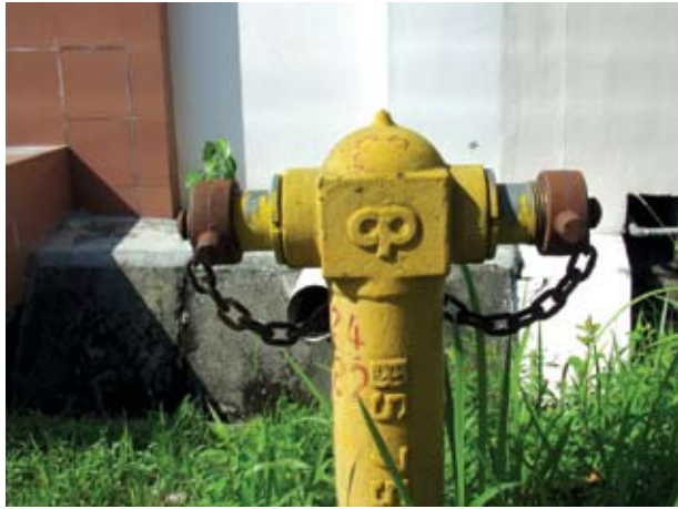
A vital fire hydrant, all parts present and correct.
