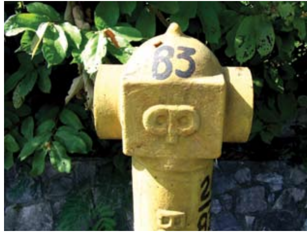
Another vital fire hydrant - vandalized by scrap thieves
