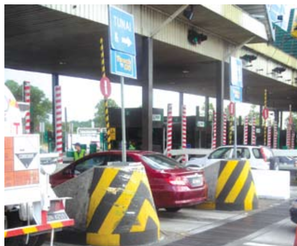
Signs of a collision at the booth.
